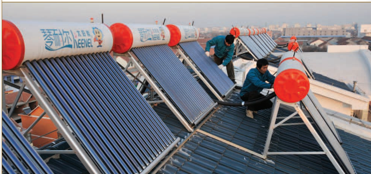
SOLAR WATER HEATERS are installed on thousands of rooftops in Rizhao, China, reducing electricity demand for domestic hot water.
